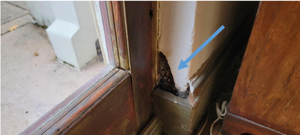
Some water damaged plaster walls (see above).
