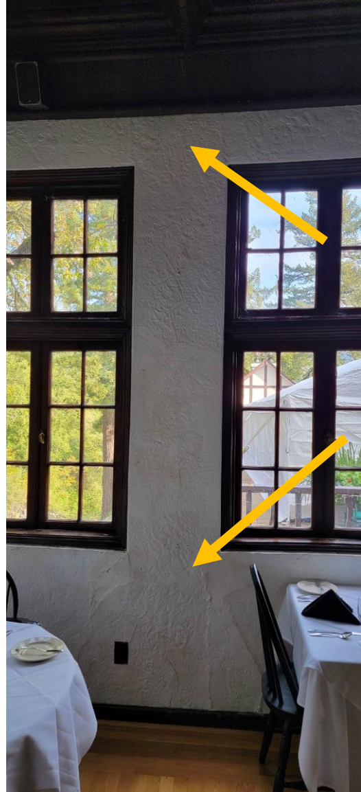
Dining inside water damage
