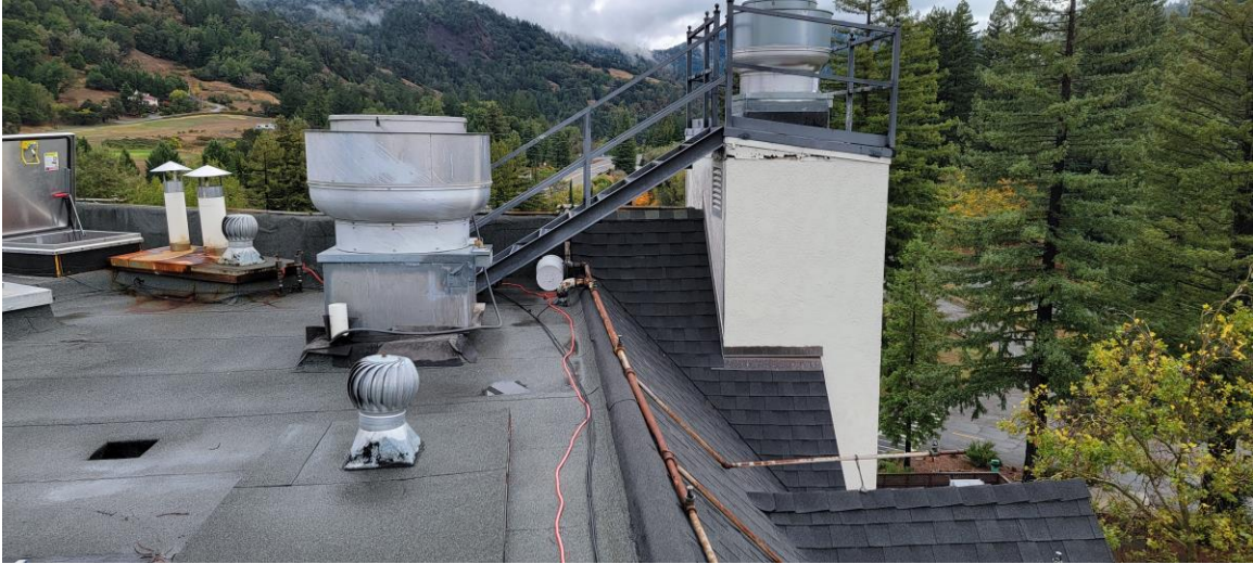
Hood Exhaust Blower Units
