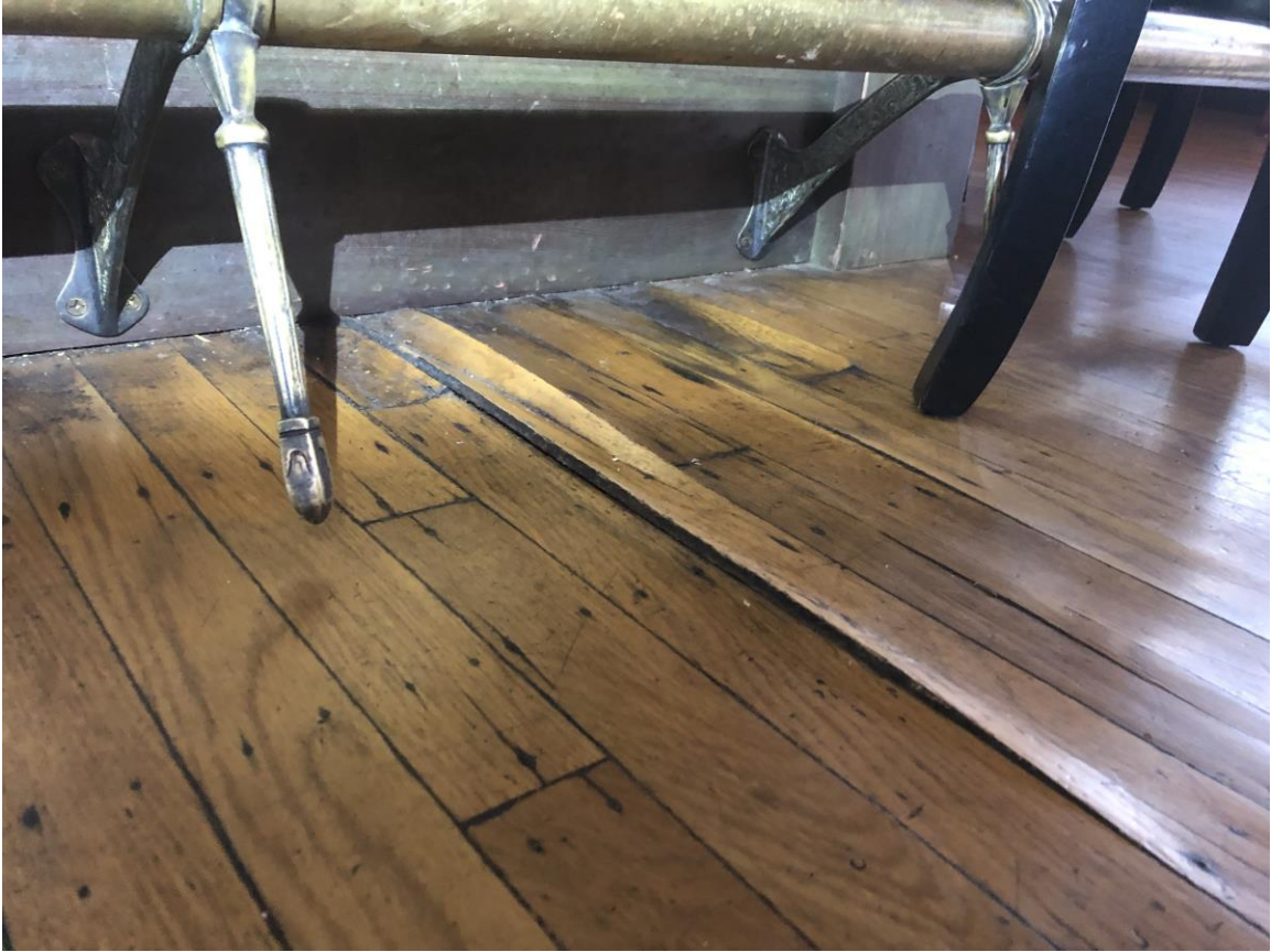
Water Damage at the Bar
