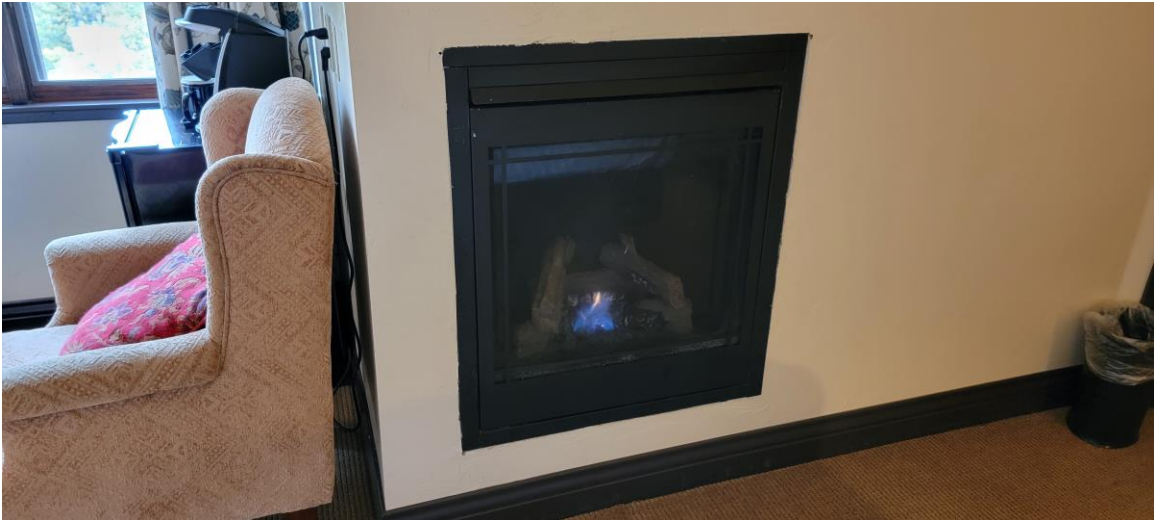
Room 406 Gas Fired Stove.
