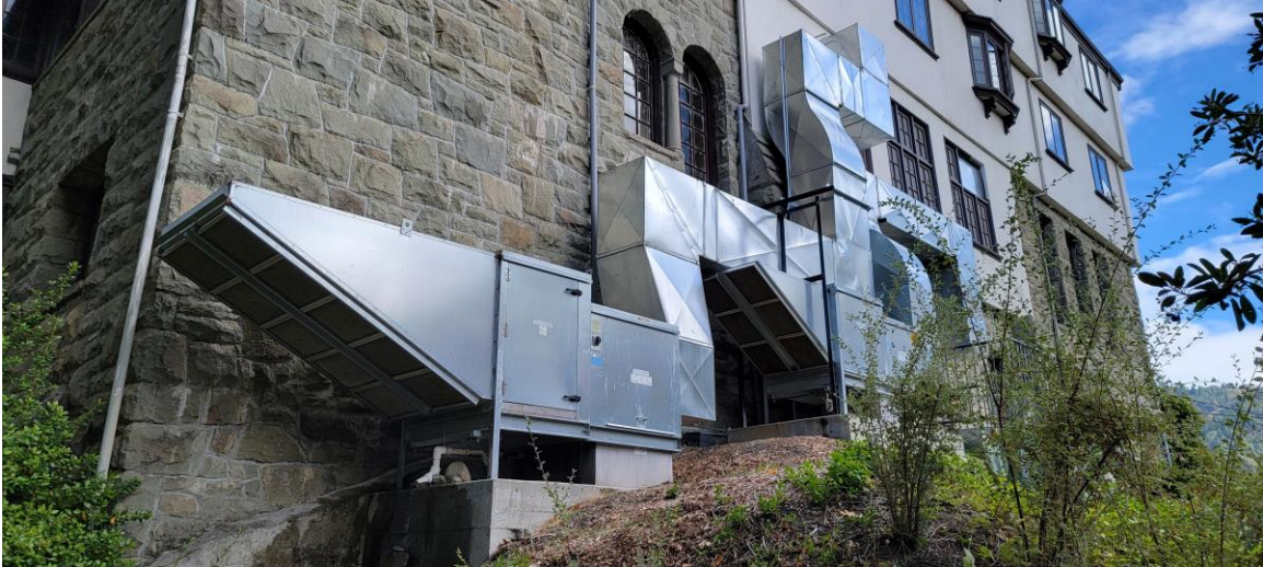
Air Intake Units Both Kitchens
